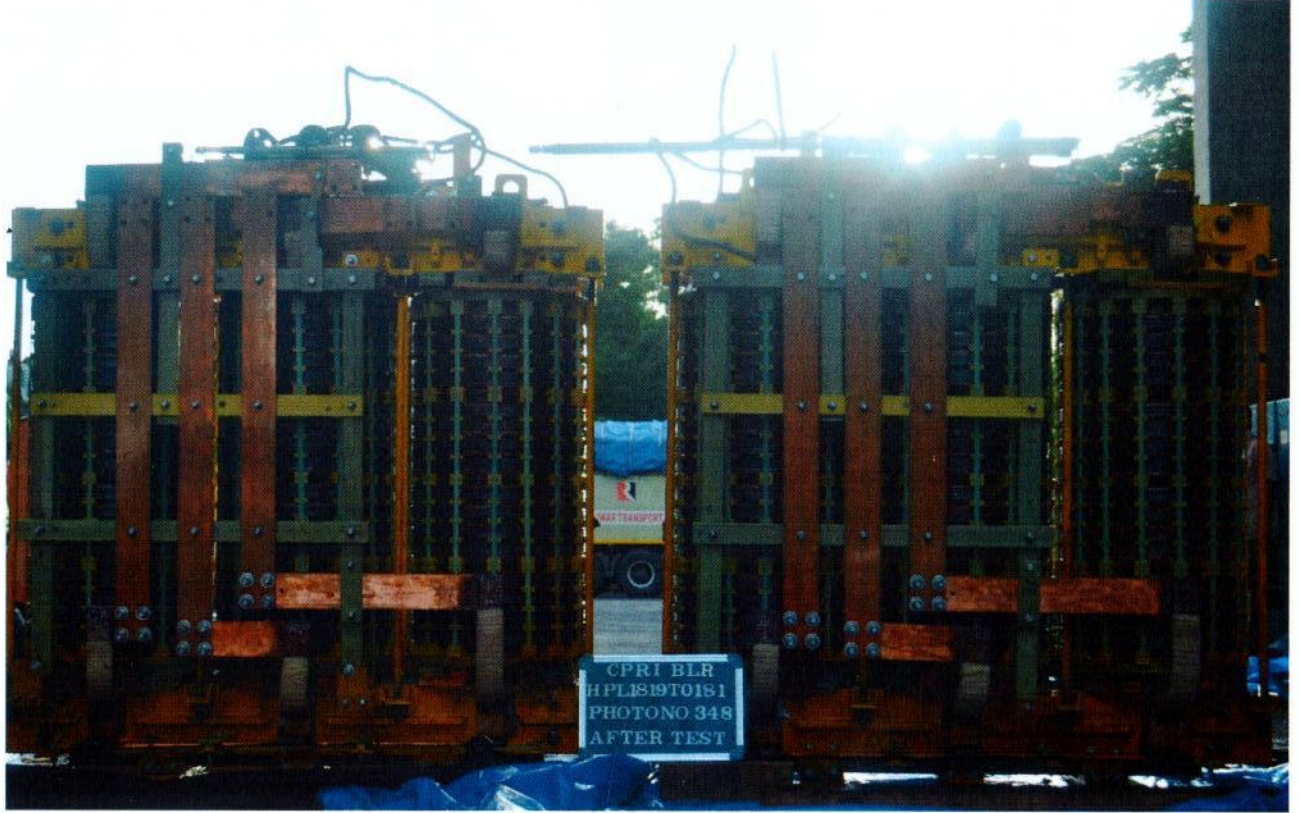
Photograph No. 348: Condition of conductor, core etc., after short circuit test, View from LV terminal side
