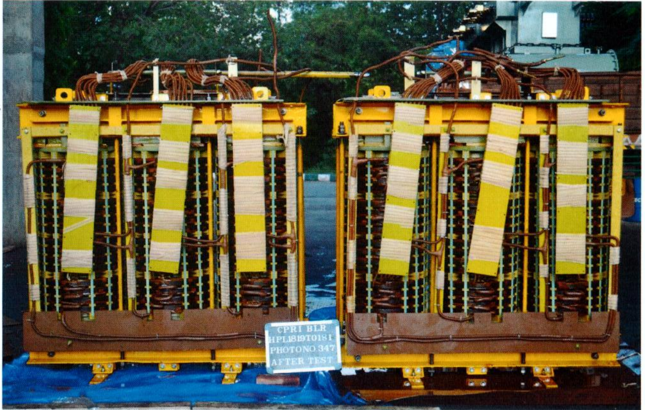
Photograph No. 347: Condition of conductor, core etc., after short circuit test, View from HV terminal side
